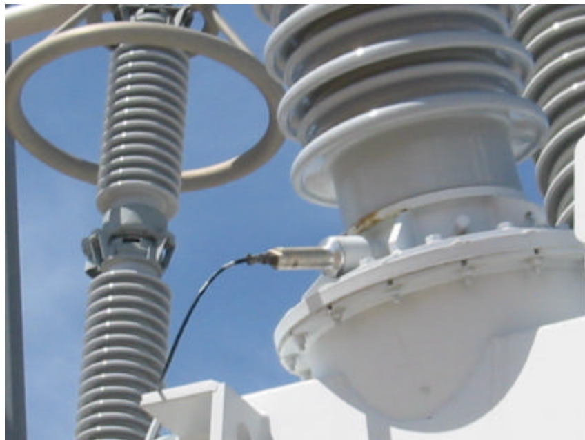
220KV bushing with a Bushing Tap Coupler (BTC) installed.
